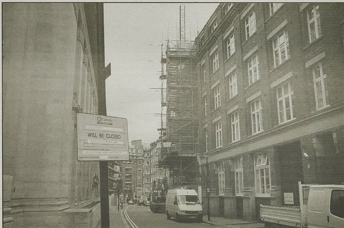
The new LSE hall of residence on Drury Lane will house 230 students. / Photo: Mark Donahue
