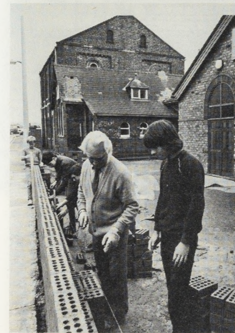
Mr Jim Ashton, senior supervisor at Ince Methodist YTS, with trainees building a new wall in front of the church.
