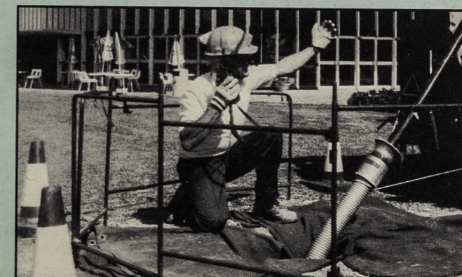
British Telecom cable being installed outside Chichester Festival Theatre. Privatisation of BT meant a complete change of culture.
