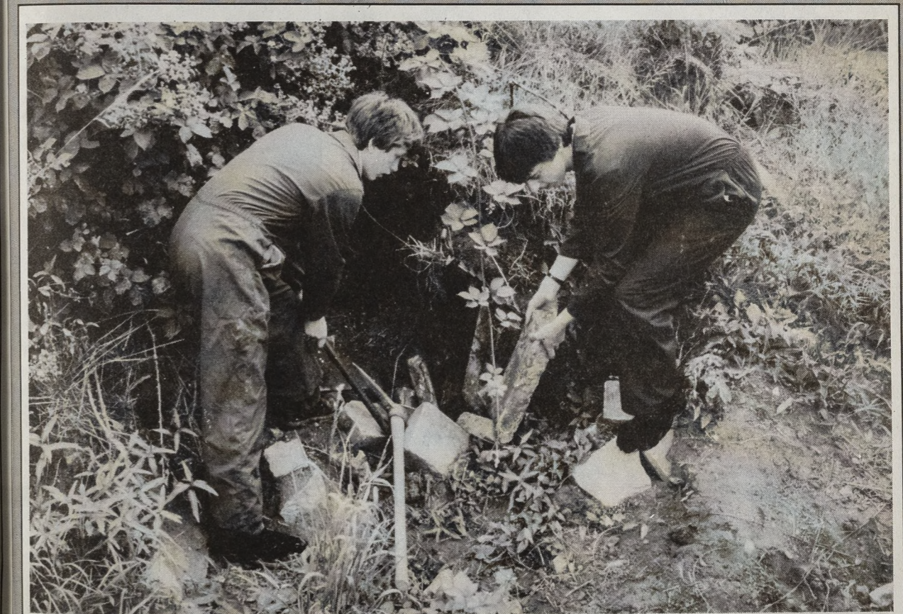
Some of the hardcore being obtained from the local authority garden centre for pier construction.
