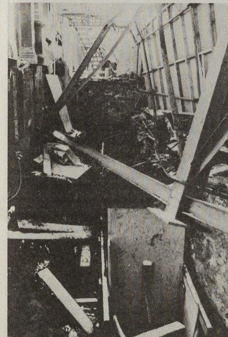
Princes Street after gantry collapsed.
