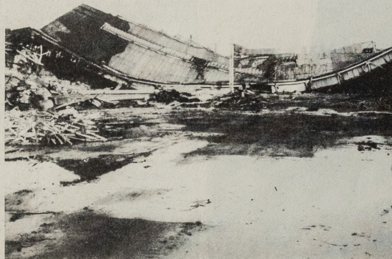
Part of the unplanned collapse of two acres of roof during demolition.
